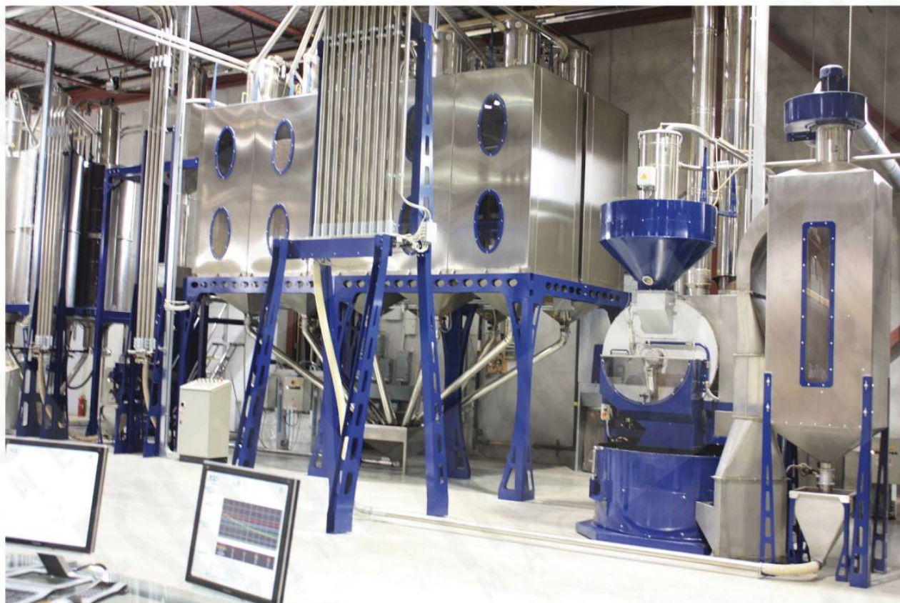
CLASSIC GOURMET COFFEE'S facility in Concord, Ontario, uses a profile roasting system that helps reduce gas consumption and CO 2 emissions by 59 percent.
